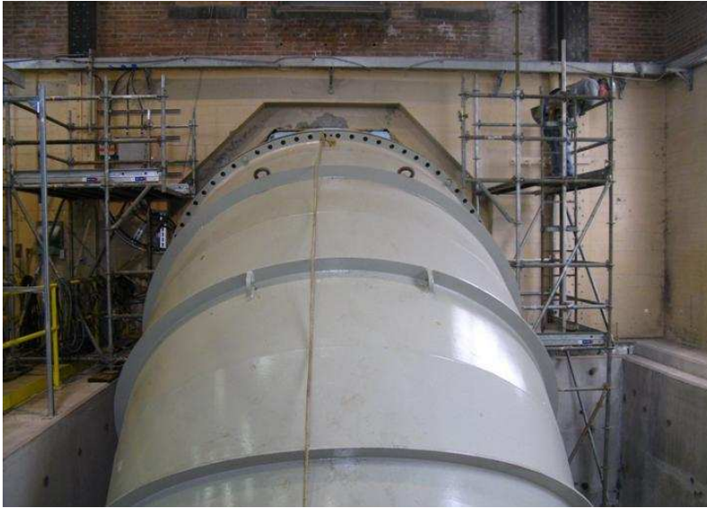
Healey Falls Generating Station Unit 1 removable steel penstock piece secured to turbine housing
