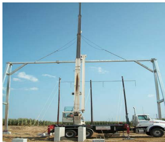
Figure 10 – Switch yard and Hydro One interconnection point. During the third quarter, Hydro One interconnection work was advancing. Market entry process and facility registration with IESO was also in progress.
