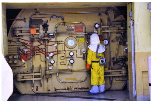
Figure 19 – A worker prepares to enter an equipment airlock that provides access to the reactor vault's interior. Restorations were recently declared complete on all airlocks and transfer chambers in unit 2.
