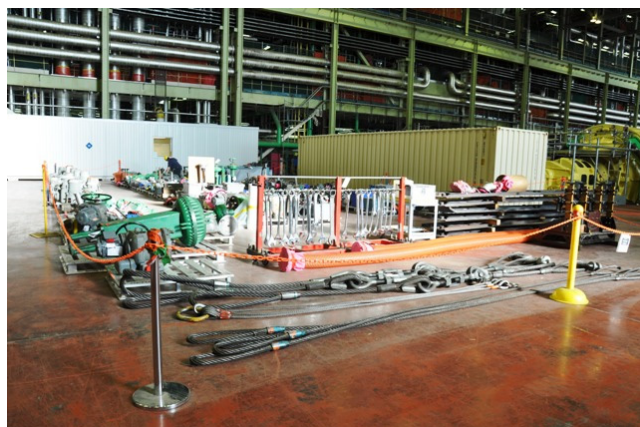
Figure 15 – Valves and their components awaiting refurbishment are staged in a lay-down area on the turbine hall floor. The valve program is more than 75 percent complete.
