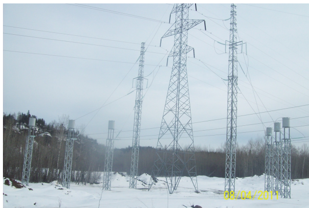
Figure 7 – A view of the Hydro One interconnection. Collection circuits were over 70 percent complete. Switching station and substation work were completed, and the project was connected as a load customer as of March 14.
