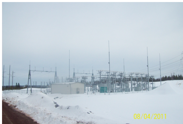
Figure 8 – A view of the substation and the control building. Hydro One completed its work in early March. At the end of the first quarter 2011, 90 percent of turbine foundations were completed. The site is getting ready to receive turbines in May.
