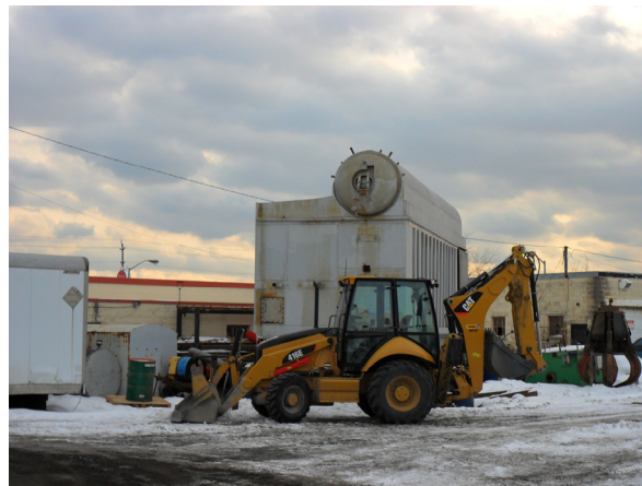
Figure 2 – A view of a boiler on-site. During the first quarter 2011, the CIA was completed and procurement activities are ongoing.
