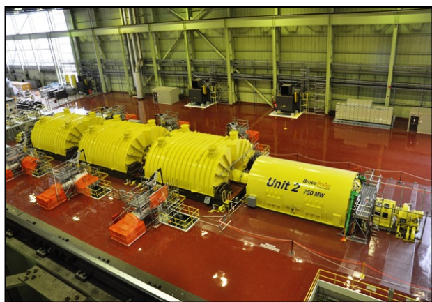
Figure 15 – Equipment and floors in Unit 2 have received a new paint job in preparation for return to service.
