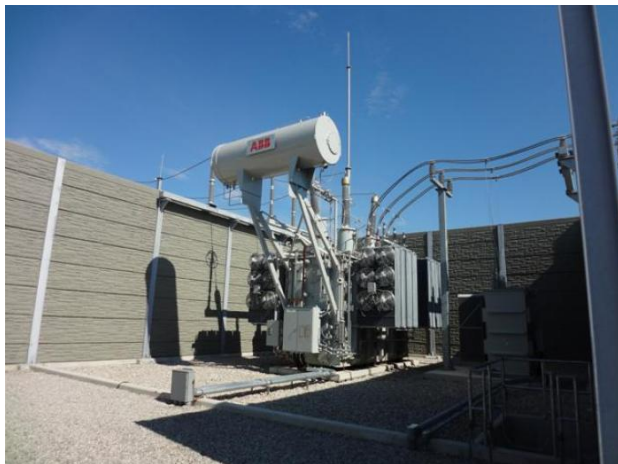
Figure 1 – Completed substation connected to the transmission system and energized.
