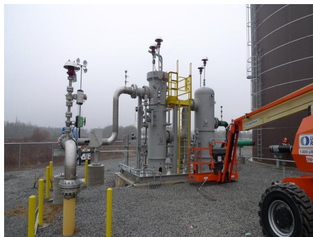
Figure 6: Fuel gas conditioning is complete. The fuel gas pipeline installation is also complete and ready to deliver gas as necessary.
