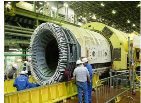
Photo 4 – The inspection of Unit 2 generator after malfunction occurred.
