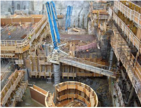
Photo 13 – A westerly view from the service bay.
