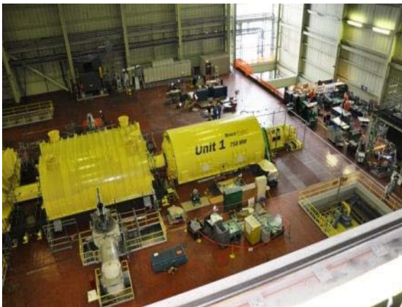
Photo 3 – The Unit 1 generator recently received a new paint job in preparation for return to service.
