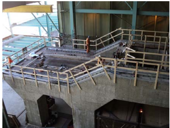
Photo 12 – A view of the condensing turbine electrical annex.
