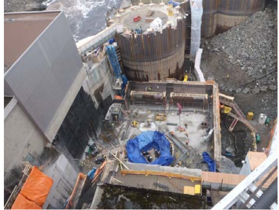
Photo 8 – A view of significant progress was made on concrete work in the intake and powerhouse prior to a failure of a temporary water retaining structure (cofferdam) before the December holidays
