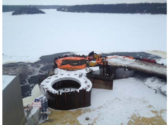
Photo 8 – Temporary water retaining structure (cofferdam) failed in December 2012 and activities for stabilizing concrete cap for cell 3 were in progress
