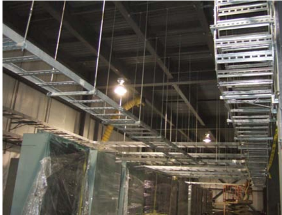
Photo 3 – Electrical switchgear and cable trays were installed
