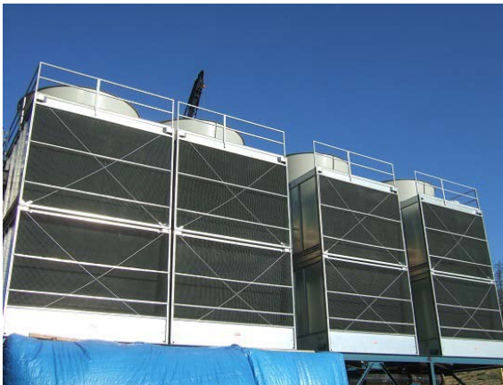
Photo 3 – Cooling tower was ready for commissioning
