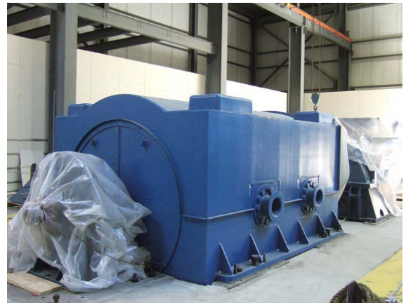
Photo 4 – Generator and turbine were in place
