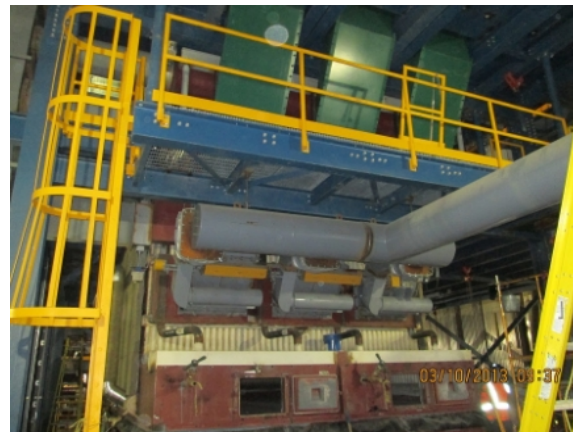
Photo 4 – Bark in-feed chutes installed on boiler
