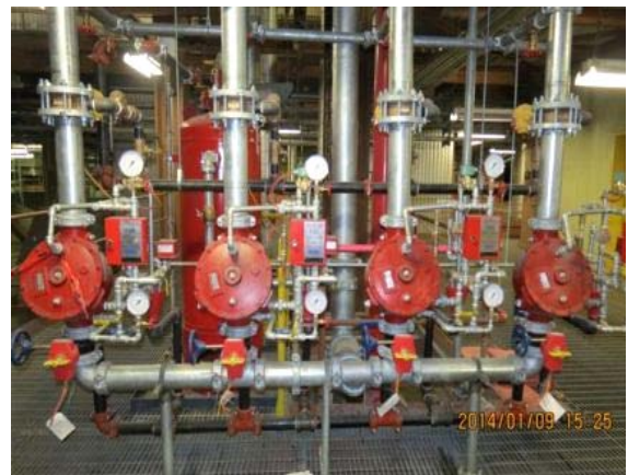
Photo 4 – View of assembled boiler system components
