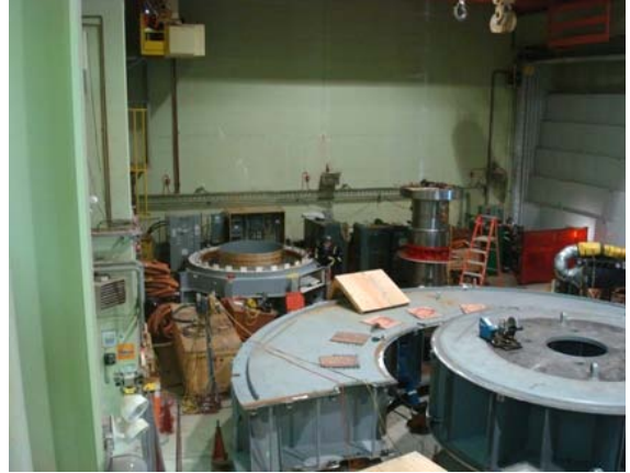
Photo 16 – Rotor assembly in the service bay
