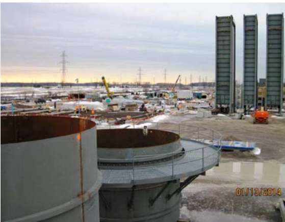
Photo 15 – View of the casing and stack assemblies for the heat-recovery steam generator
