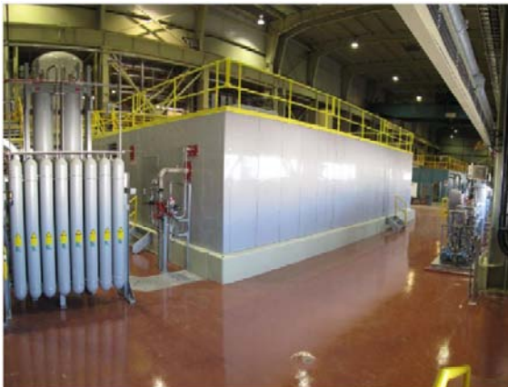
Photo 19 – View of the facility now in commercial operation
