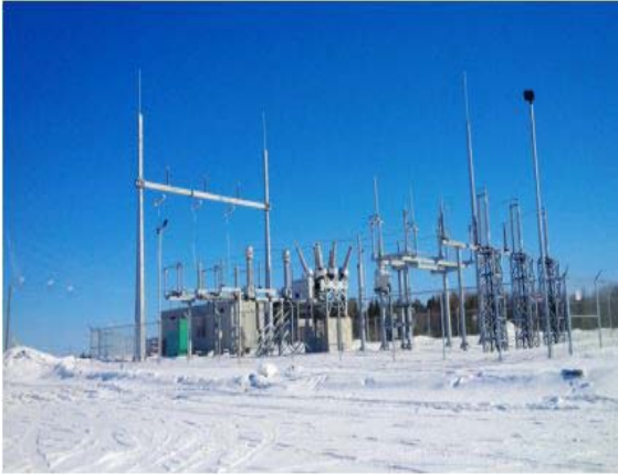
Photo 21 – Switchyard emergency diesel generator set on pad
