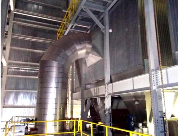
Photo 9 – Internal view: bag house outlet duct
