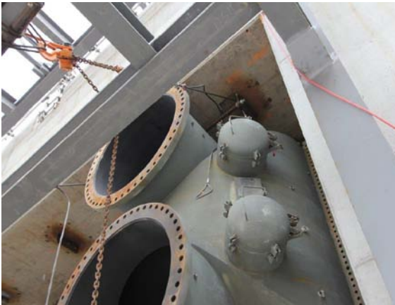
Photo 11 – View of the base of the heat recovery system
