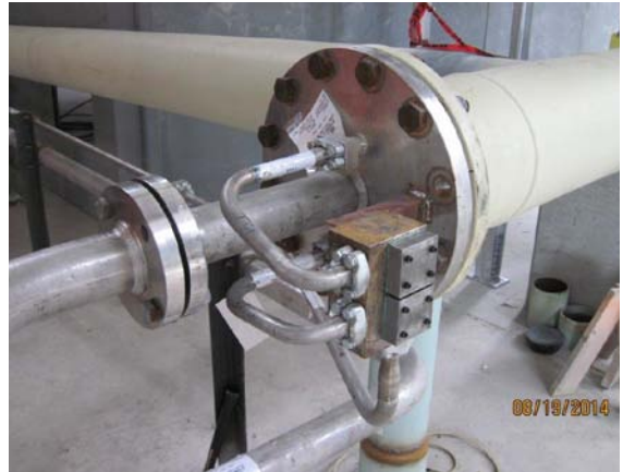
Photo 12 – Internal view of the facility: pipelines and flange
