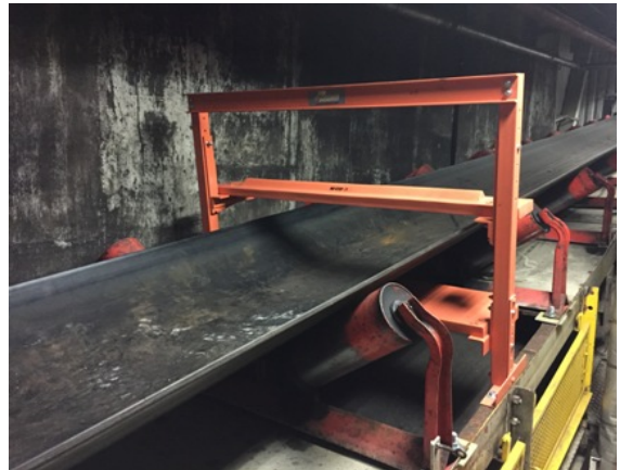
Photo 22 – Metal detector installed
