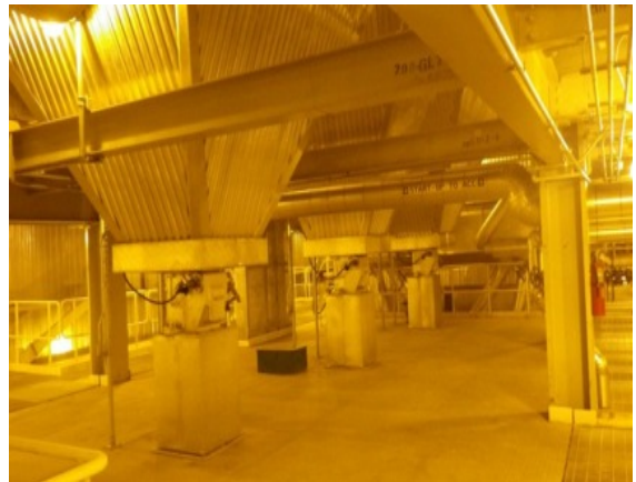
Photo 4 – View of convection pass fly ash hoppers
