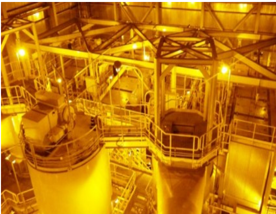
Photo 3 – Internal view of lime silos and bag houses
