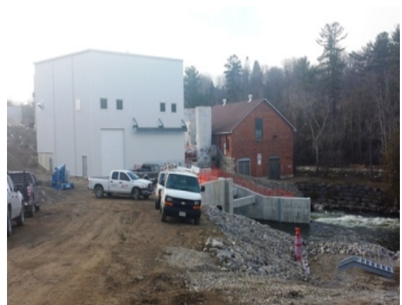
Photo 19 – View of the new powerhouse
