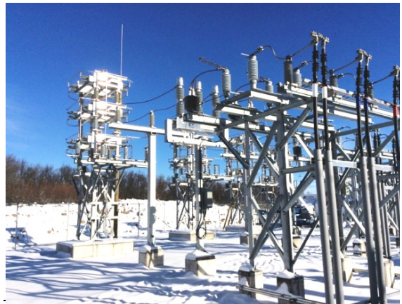
Photo 8 – Switch yard connected to the solar farm
