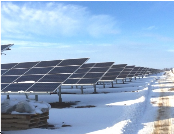
Photo 7 – Solar panel array
