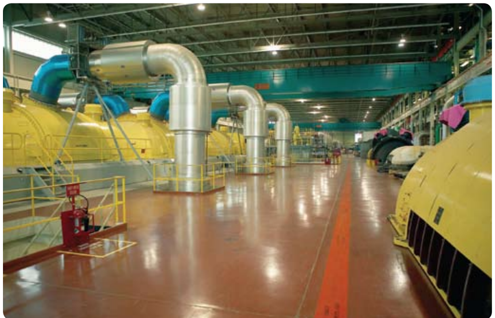
Pickering A, Unit 4, Turbine Hall
