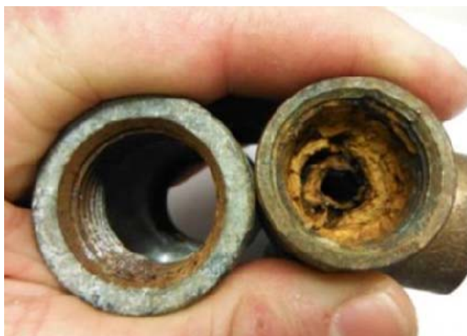
Figure 1. On the left is a clean, 1 inch diameter galvanized water pipe while on the right is a clogged pipe of the same diameter which has water flow restricted to approximately 25% or the original diameter.
