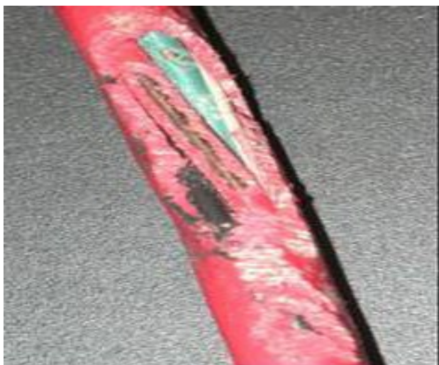
Figure 1. Signs of chewing on electrical wire
