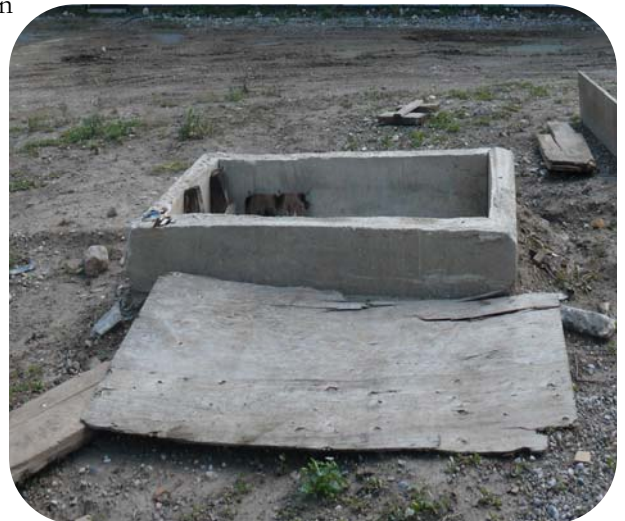
Photo 1. Fosse de visite
