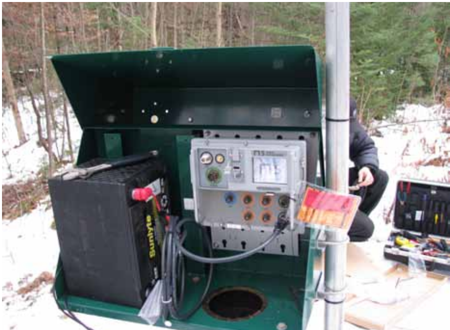
Inside one of Quinte Conservation's groundwater monitoring stations.
