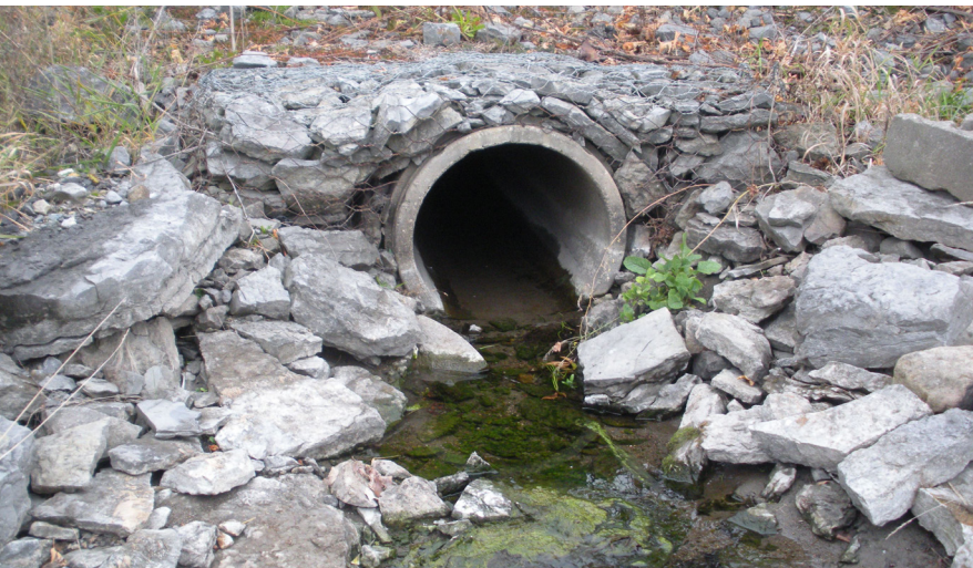
A Stormwater drain with contaminated water.
