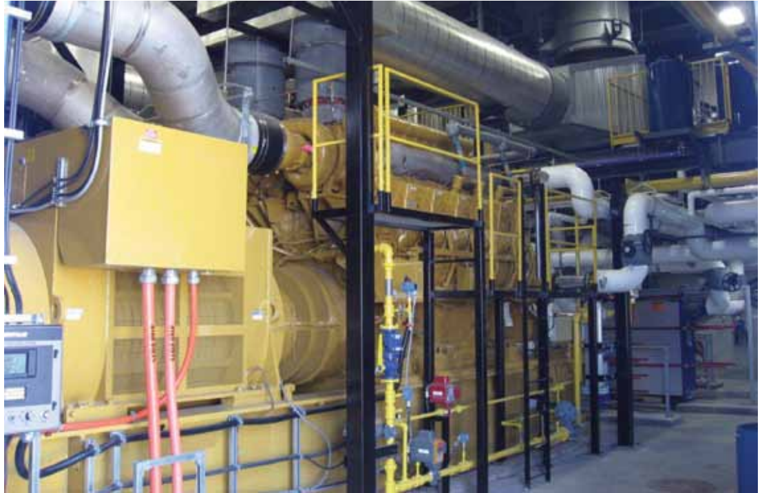
Photo : Markham District Energy Inc.
