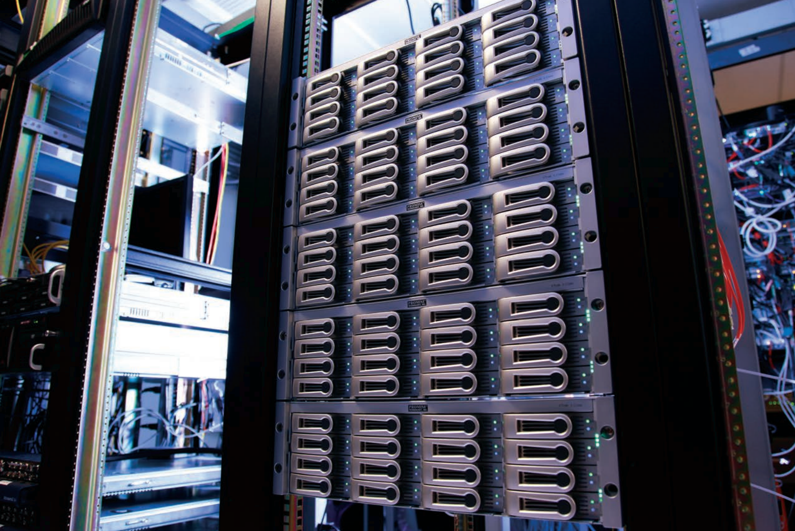
TFO's Storage Area Network (SAN) production server
