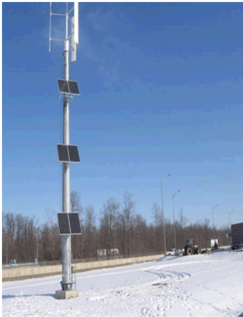
6 kW Windmill -Solar device at Sarnia TIS
