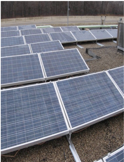
10 kW Solar device at Windsor TIS
