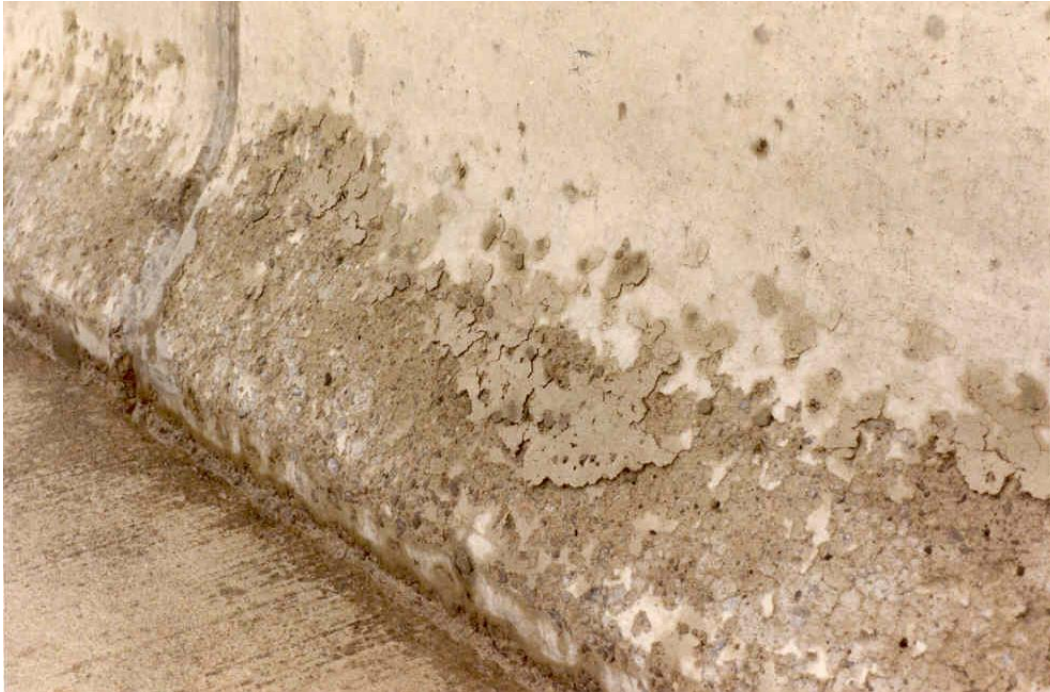
FIGURE 5 Example of Severe Scaling
