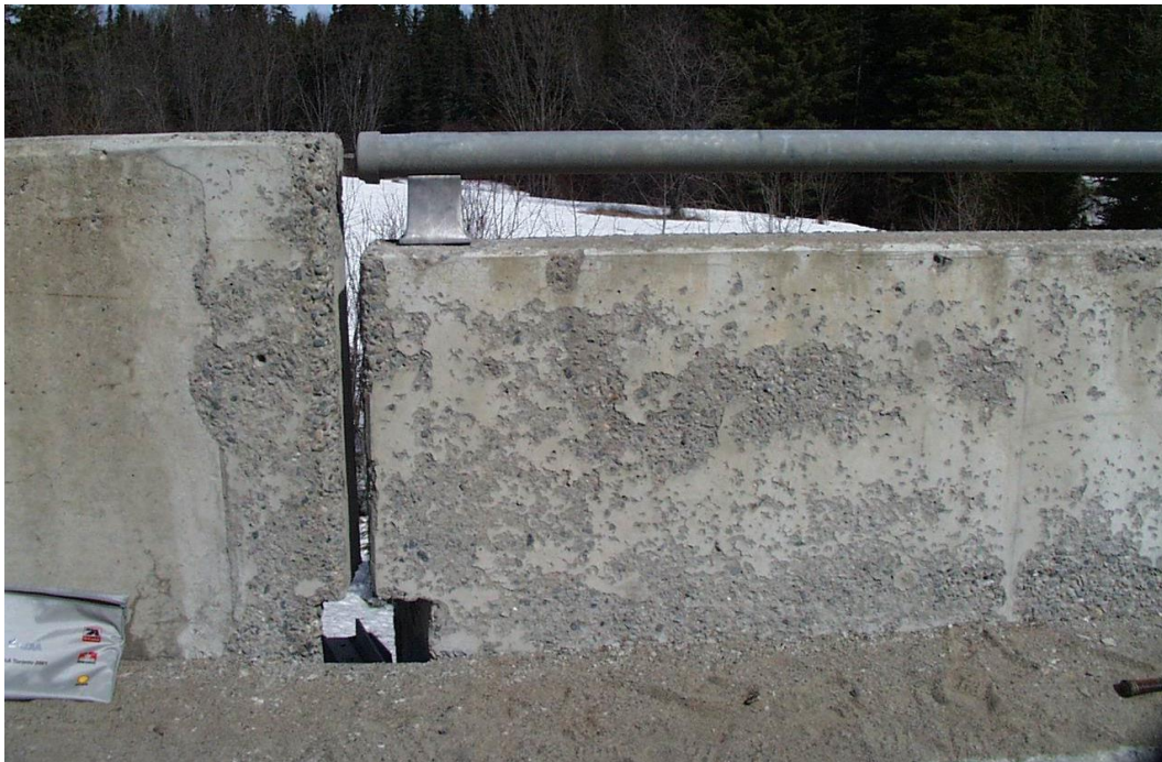
FIGURE 6 Example of Severe Scaling
