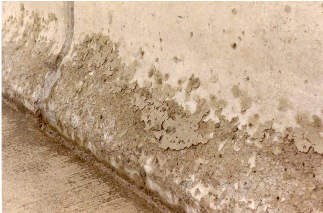
FIGURE 5 Example of Severe Scaling
