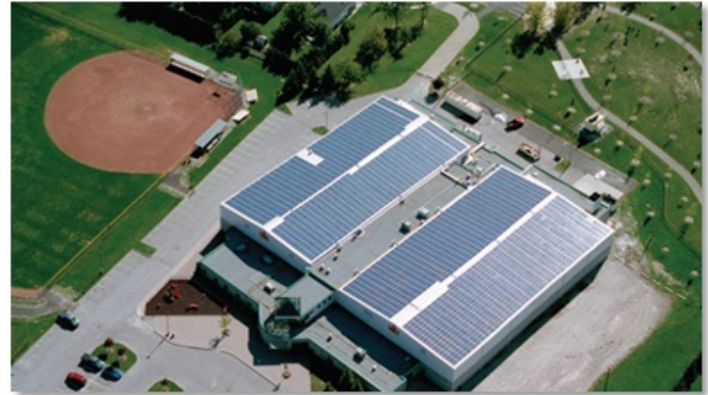
FIT 1 rooftop solar (PV) project (500 kW), Tecumseh, ON
