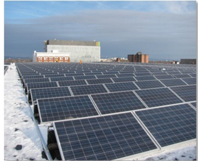
FIT 1 rooftop solar (PV) project (280 kW), Thunder Bay, ON
