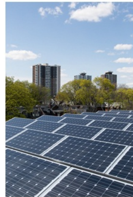
FIT 1 rooftop solar (PV) project (23kW) Toronto, ON
