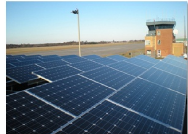
microFIT rooftop solar (PV) project ( \leq 10 kW), Kingston, ON
