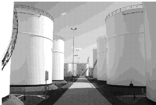
PHOTO: TANK STORAGE FACILITY AT KOOLE'S ROTTERDAM TERMINAL.
