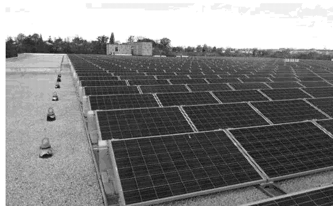
Commercial rooftop solar array.
