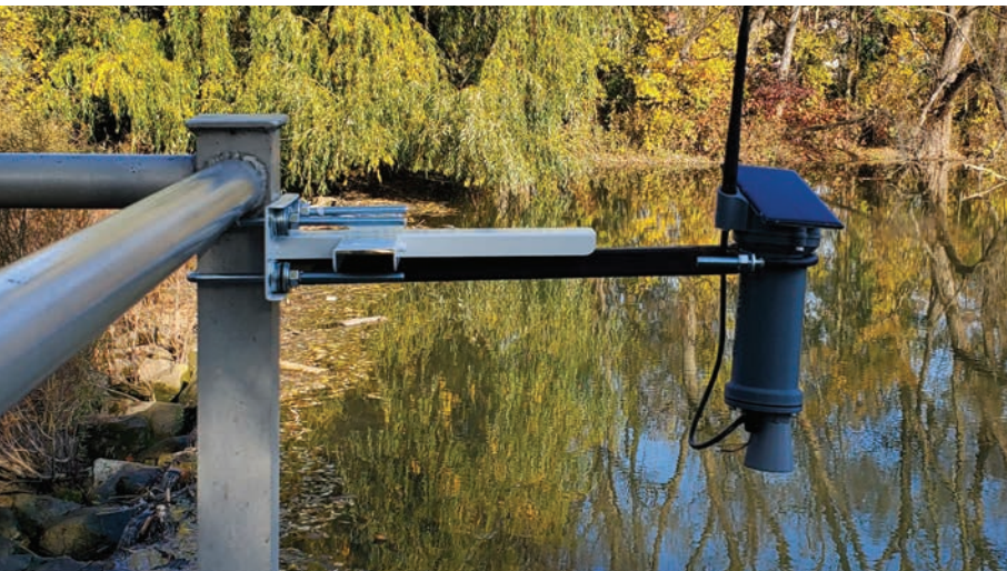
New water level sensor installed at the Head Street Dam in Strathroy.
