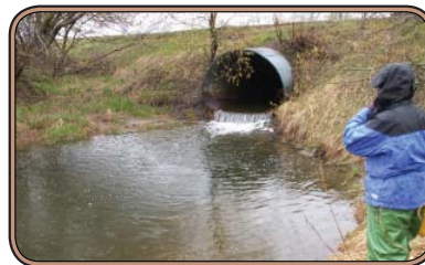
Stark Drain prior to remediation.
