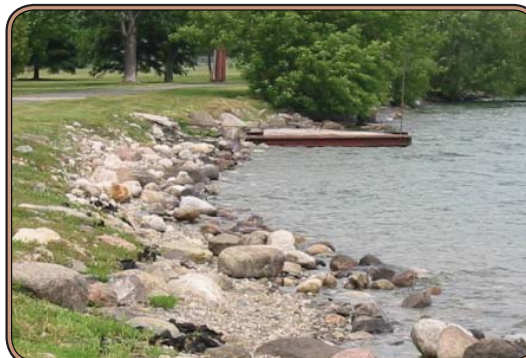
Morrisburg shoreline prior to erosion repair.
