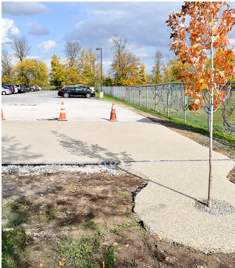
LID demonstration site at SNC's Administration Office
