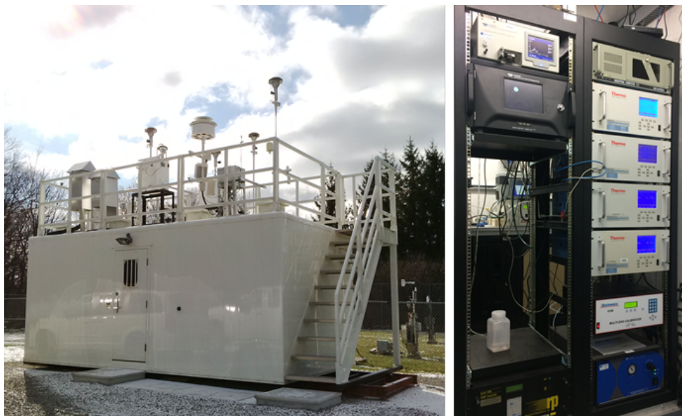
Two photographs showing the exterior (left) and interior (right) of the Toronto North Air Quality Health Index Station.
