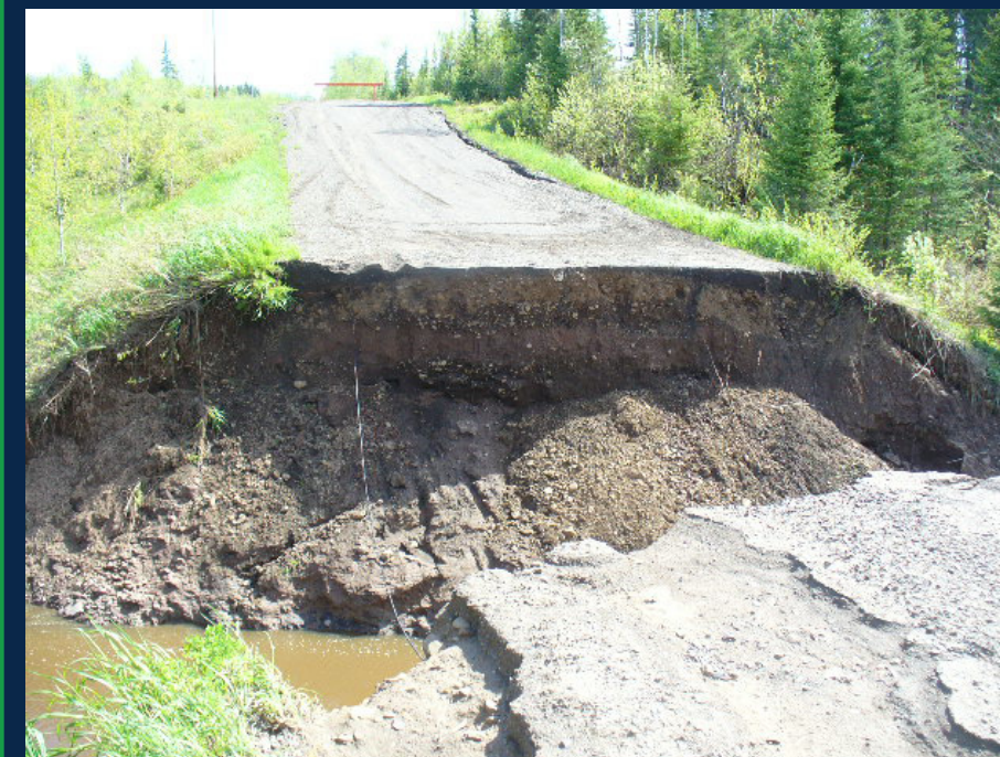
Damage caused by flooding in 2008.
