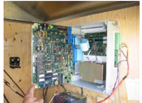
The Chatham Water Level Gauging Station is equipped with enough instrumentation to measure water level, water and air temperature, as well a weighing type precipitation gauge that measures rain and snow. The entire station, as well as the pressure transducer that measures water level, is powered by a solar panel. Above is the instrument that stores the data for downloading.
