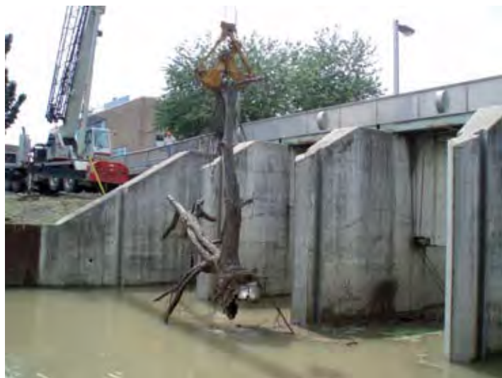
The McGregor Creek Dam is used to prevent high Thames River water from entering the south Chatham area. Under normal flows while the dam is open, debris such as this log can accumulate upstream of the dam. The debris must be removed in order for the dam to operate effectively.
