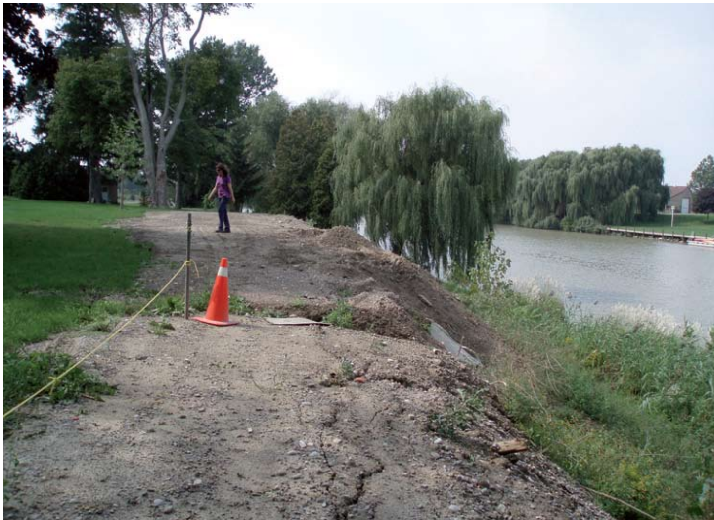
One of the purposes of the Conservation Authority Regulation is to ensure fill is placed such that banks remain stable and that a watercourse's capacity is not impacted. The above area was investigated by Conservation Authority staff in 2011.
