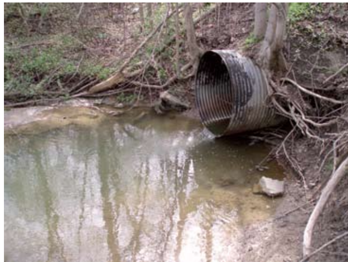
This perched road pipe culvert is a blockage to fish migration upstream. The Conservation Authority, DFO and municipalities work together to achieve a solution that benefits all. The pipe will be extended to allow for a wider, safer top road width. Lowering the pipe outlet below the bed of the stream will allow for fish passage through the pipe to access upstream spawning areas.
