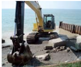
Staff investigated a complaint from a resident on Erie Shore Drive regarding a backhoe working in the water on Lake Erie, without any sediment control.
