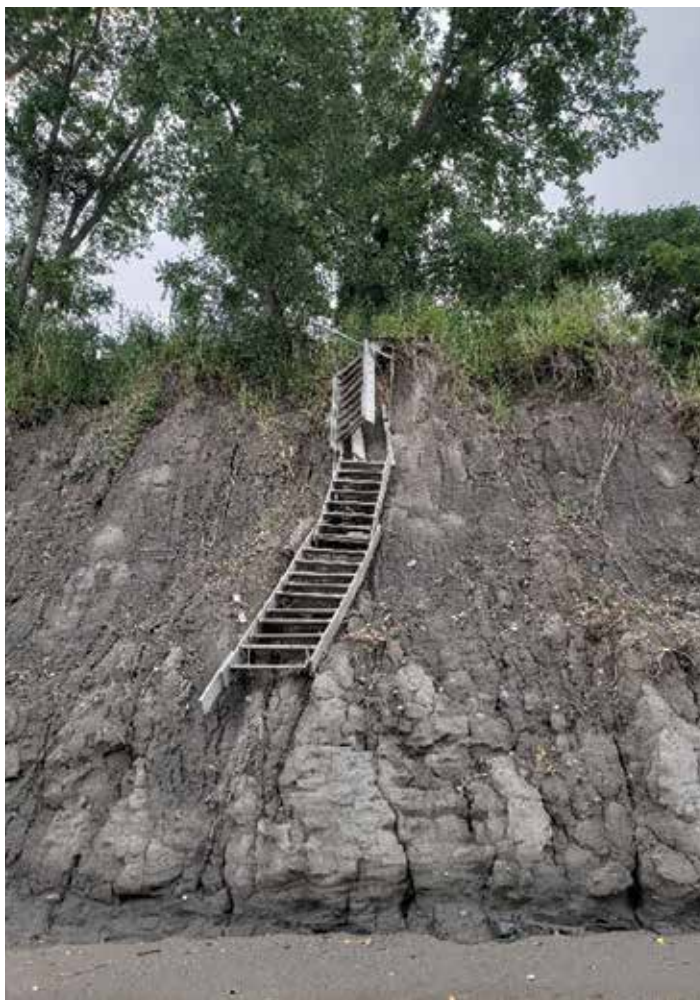
Works on eroding bluffs are not stable.
