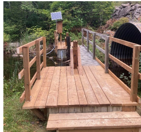
Pine Lake Dam Safety Controls
